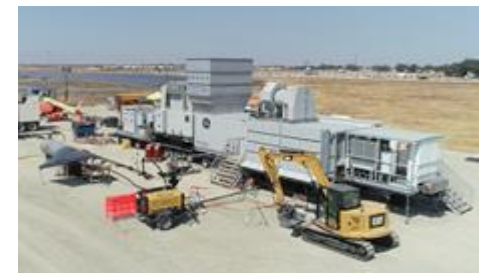
Power deployed four TM2500 aeroderivative gas turbines to support California's emergency power needs
