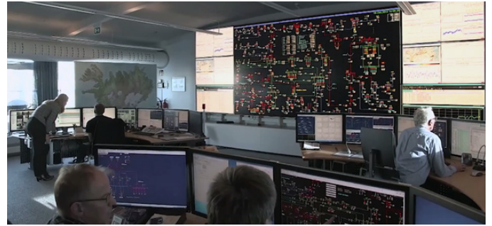
Landsnet control room, showing PhasorPoint in use.
