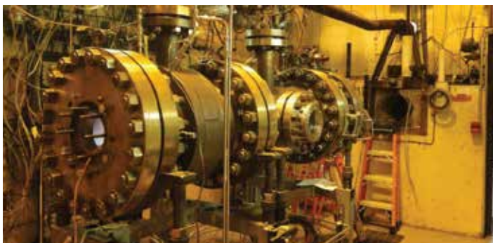
Figure 7 – Single nozzle combustor at GE Global Research's facility
