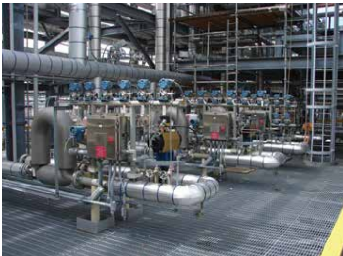
Figure 13 – Fuel blending hardware at a USA site
