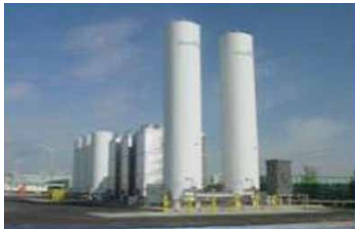
Figure 9 - Fuel blending system at GE's Gas Turbine Technology Lab
