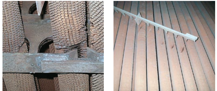
Figure 1: Fin Wear from Friction with Damaged Restraint
