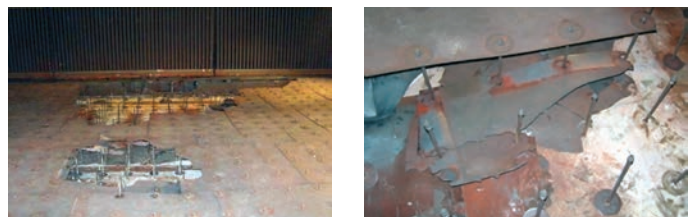
Figure 2: Damage Liner Plate and Stud Bolt from GT Strong Flow and Pulsation
