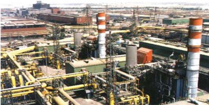
Figure 7. Gas turbine and heat recovery steam generation (HRSG) for the first GE combined cycle power plant in Italy burning BFG/COG/LDG mix.
