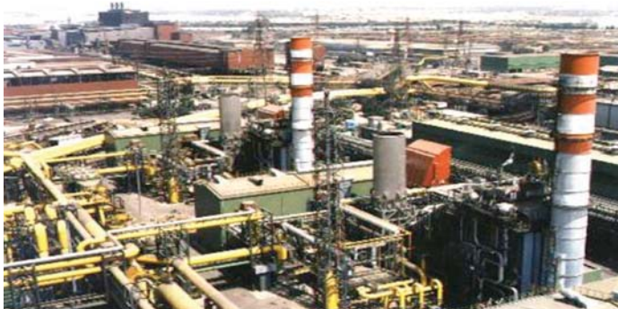
Figure 7. Gas turbine and heat recovery steam generation (HRSG) for the first GE combined cycle power plant in Italy burning BFG/COG/LDG mix.
