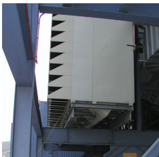
Figure 1. Gas turbine inlet with weather hoods
