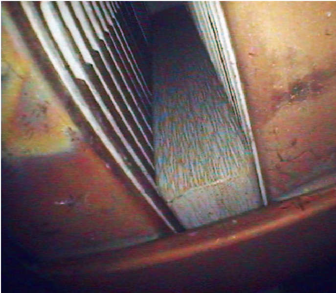
Figure 5. Field coils picture taken by borescope
