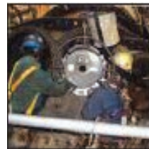
Flow Sleeve Removal
