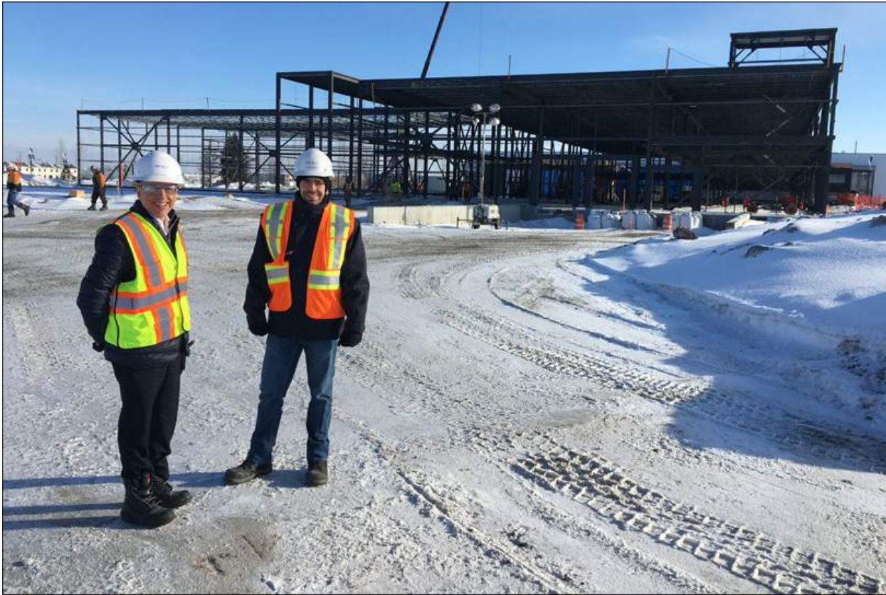
Fig. 7 Alain Dupont, President of AP&C, at the construction site of AP&C's new state-of-the-art titanium powder factory in St. Eustache, Montreal, Canada, in February
